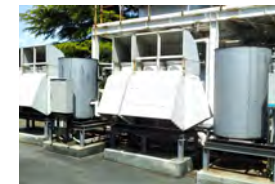
Chiller (Cooling water circulation equipment)
