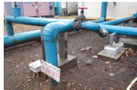
Emergency feed-water valve in Hachioji General Plant
