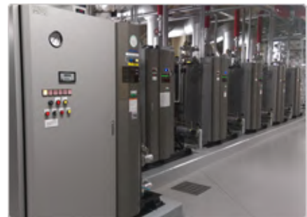
Boiler at the Kashima Pharmaceutical Plant
