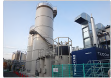
Biomass Electricity Generation at the Hachioji General Plant
