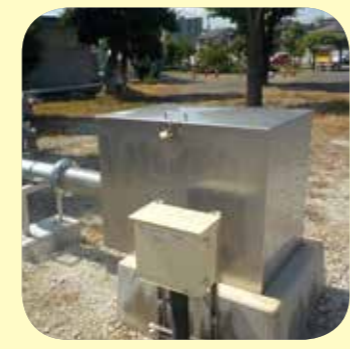
A new well was dug at the Nissui Anjo Plant. The additional well will improve water quality and reduce the number of times the filter needs to be cleaned (backwashed) after pumping up, thereby greatly reducing the amount of water used.
