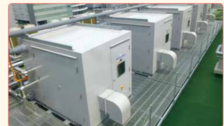
Roof-top freezing machines using the natural refrigerants ammonia and carbon dioxide
