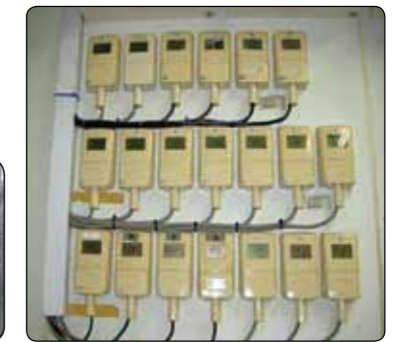
Integrating flow meters for checking the total daily water usage
