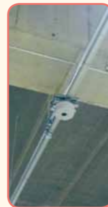
Camera installed on the ceiling inside the warehouse
