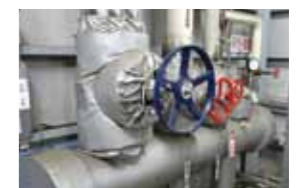
Insulation jacket can be seen attached to the blue valve
